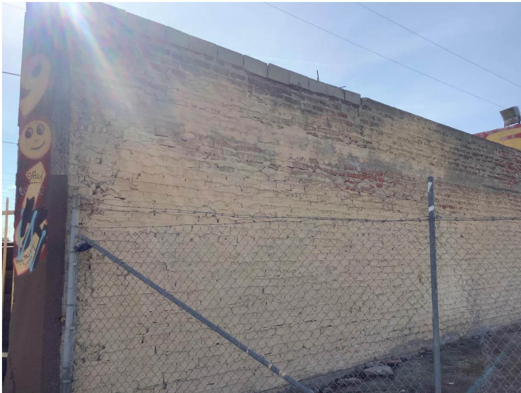
Figure 5-4. Overview of rear of tire shop at eastern edge of tire shop property, facing southwest.
