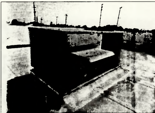
Split rooftop units serving credit union
